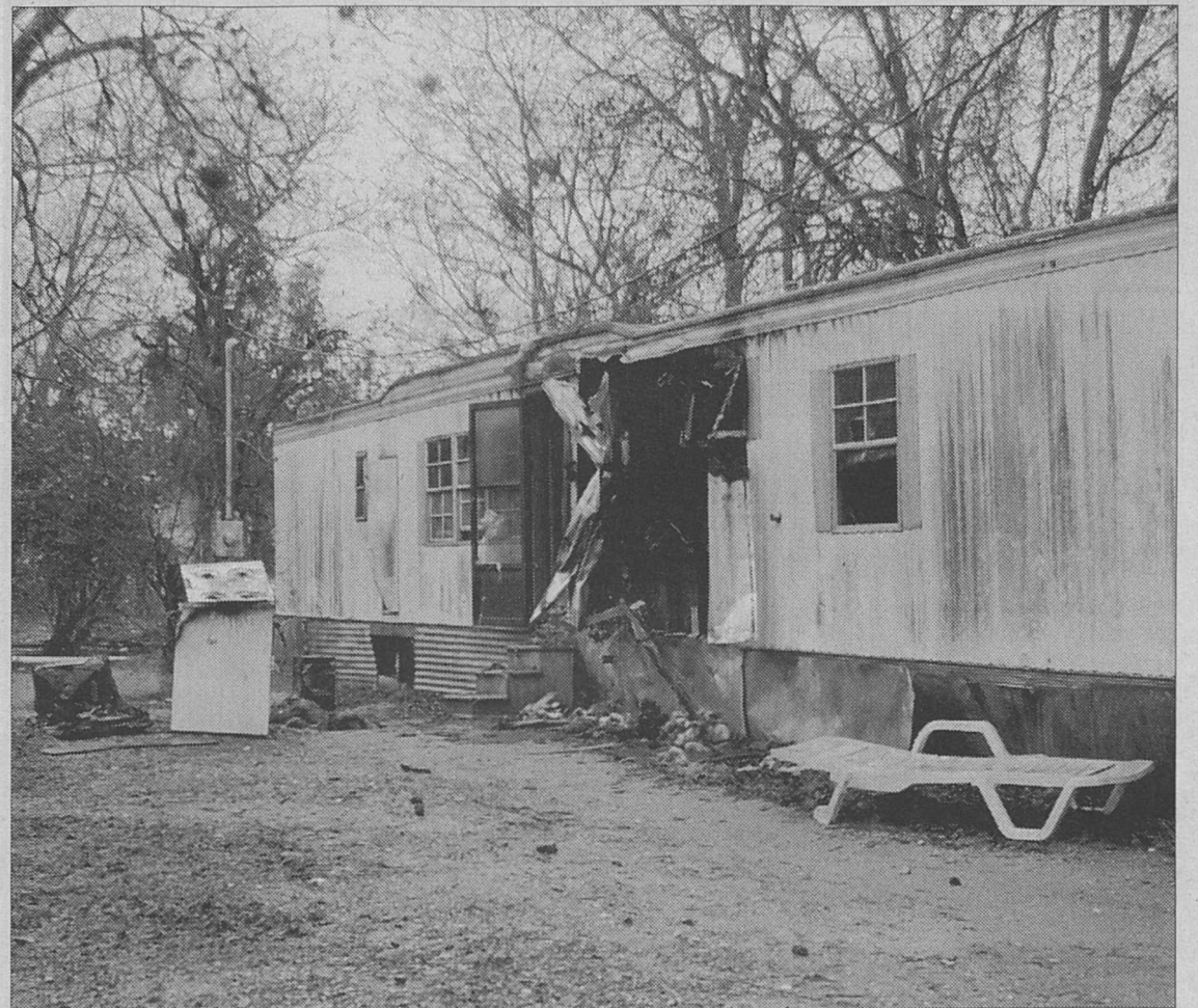
At 11:48 pm, on Saturday, Dec. 23, Sgt. David Weise assisted the Eagle Lake Volunteer Fire Department in the 400 block of Second St. with a mobile home that was on fire. It was determined that the fire started due to faulty electrical wiring.
